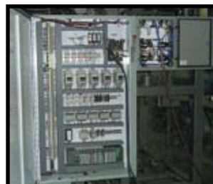
Standard Electrical Panel
