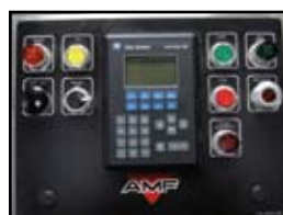
Operator Interface Panel
